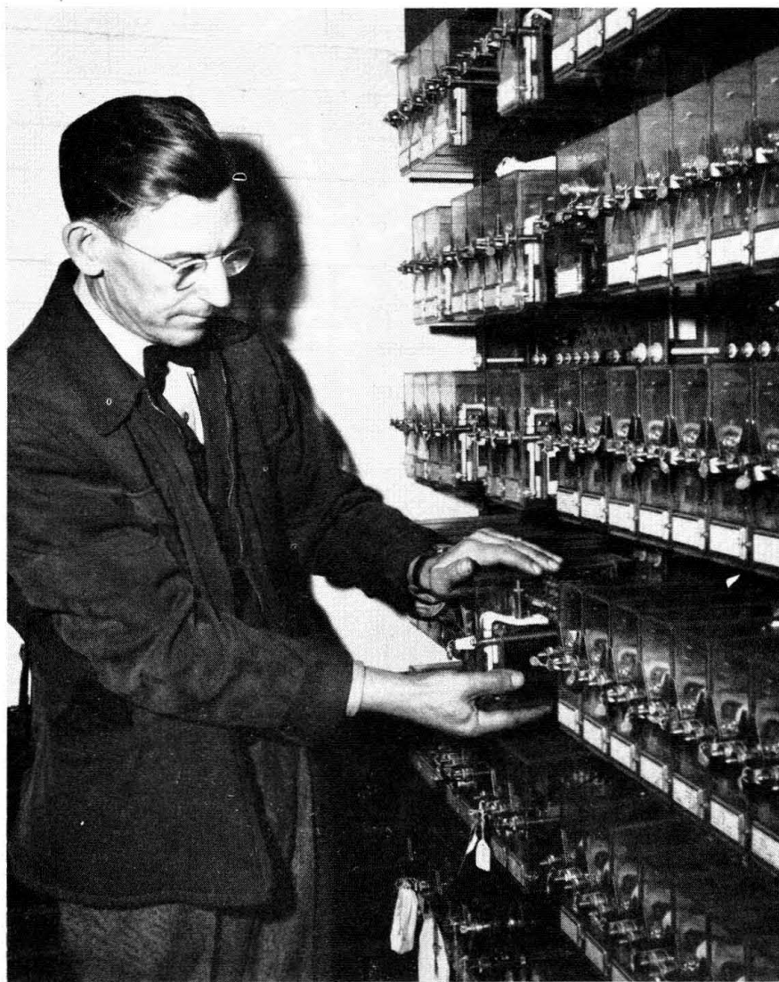
There are 1,511 Type-B relays on this installation—935 in the tower, and 576 in the field
