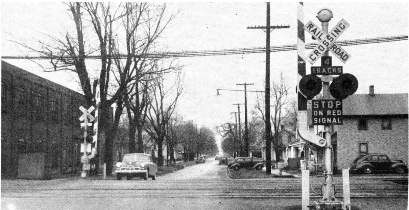
As part of the project, new highway crossing protection was installed at several crossings in the vicinity of the plant
