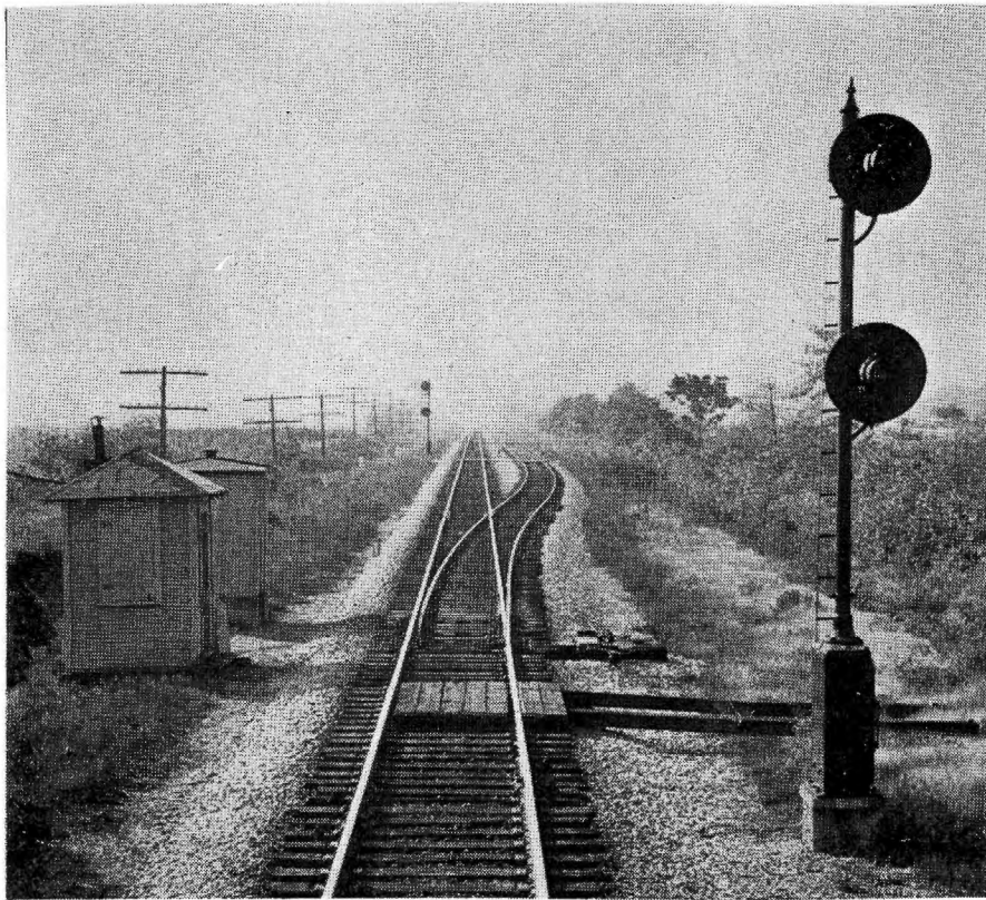
The new longer sidings are equipped with power switch machines and searchlight signals controlled by the C.T.C.
