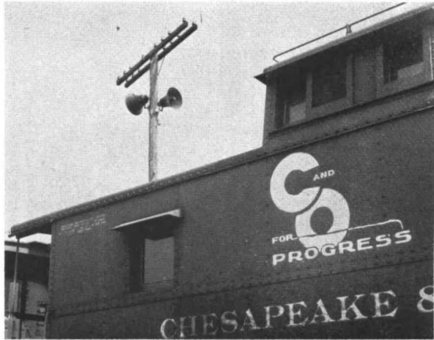
Paging speakers mounted high above ground to provide coverage over several tracks
