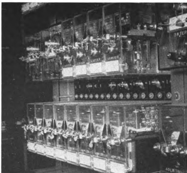
Plug-in relays used extensively at instrument housings
