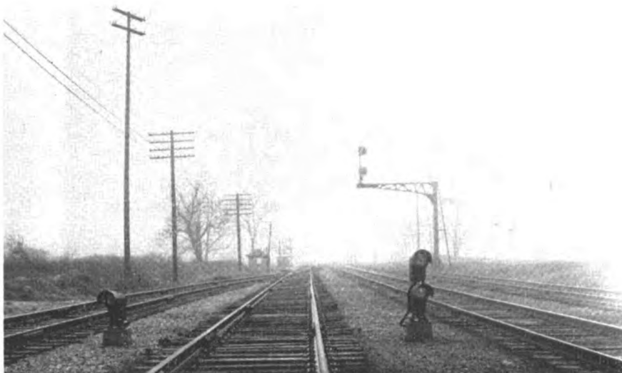
Signals R37 (dwarf) and R39 (cantilever) looking towards yard entrance
