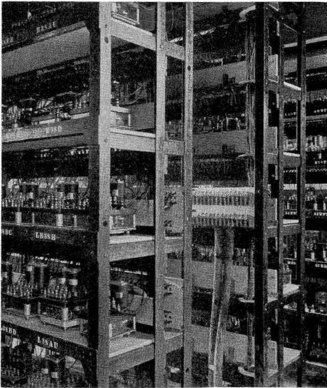
Relay racks in tower constructed of asbestos board on angle iron
