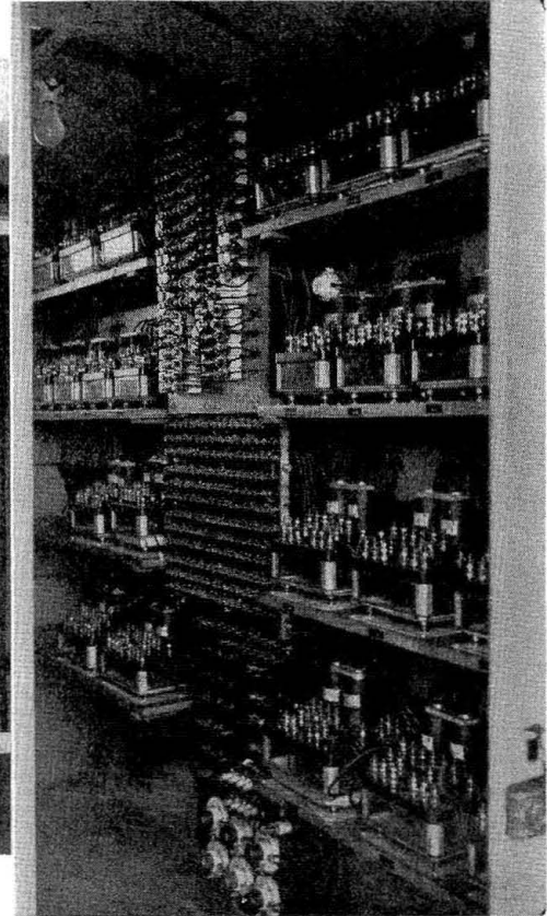
Interior of sheet metal instrument housing
