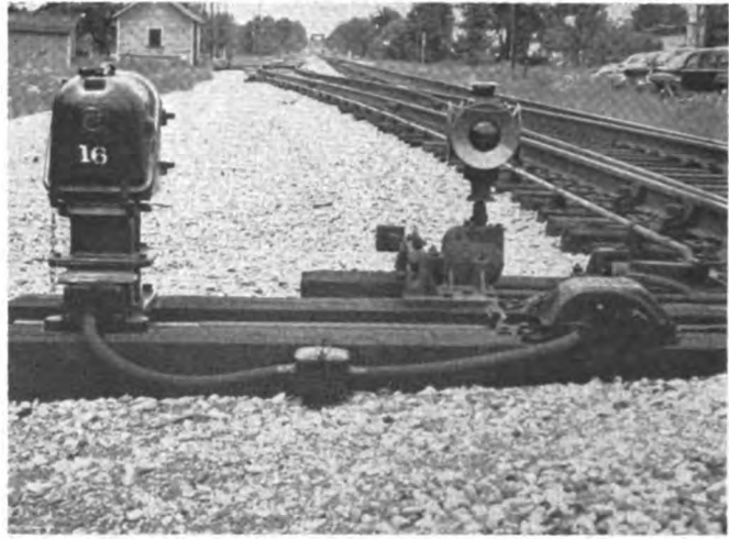
HAND-THROW SWITCHES are equipped with electric locks
