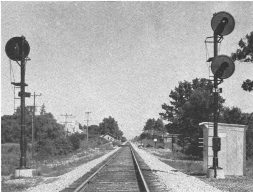
A sheet-metal house, instead of cases, is used at intermediate signals so that relays and battery are not exposed to rain during inspections
